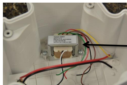
Back Can With R70VT Transformer Installed
